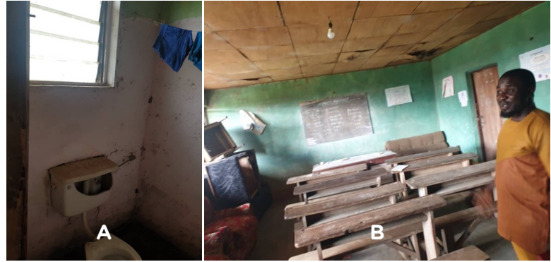
Fig 3 . Need assessment visit to Tombel MYEC A: an old abandoned toilet and B: The general hall with broken furniture
